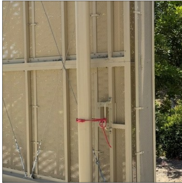
[Gate involved in incident]
