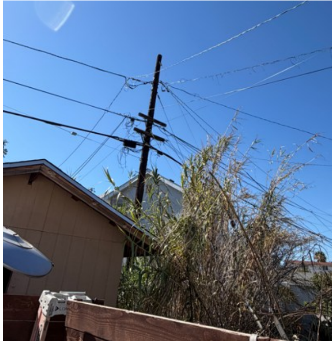
[Electric incident resulting in fire damage]
