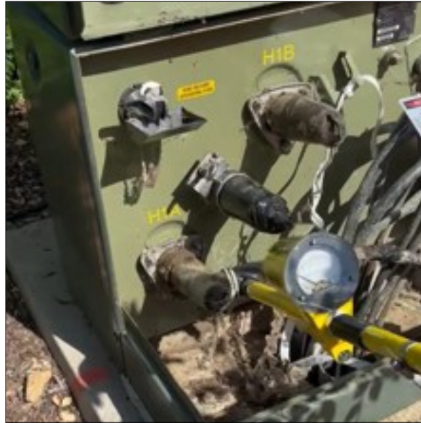
Testing for voltage with the volt meter at the transformer in question
